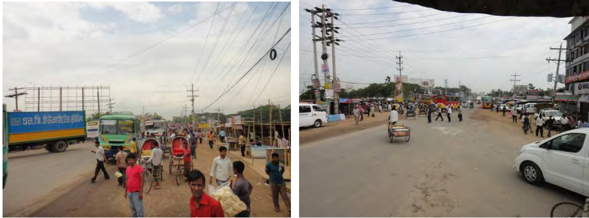
Figure 11.2: Criss-crossed Overhead Electric Lines
